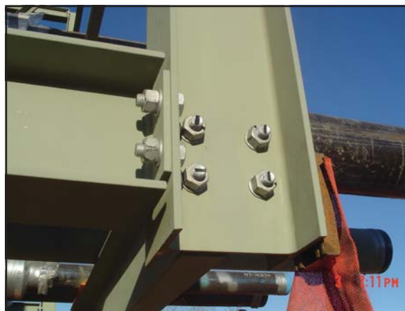
What turn was put on these bolts?
