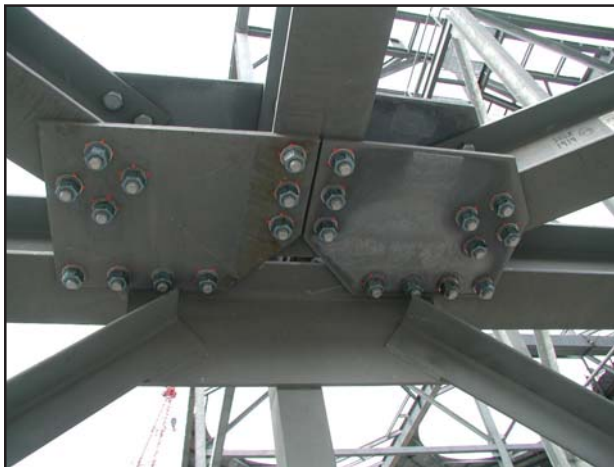
Figure 1: Squirter DTIs came out of construction concerns
